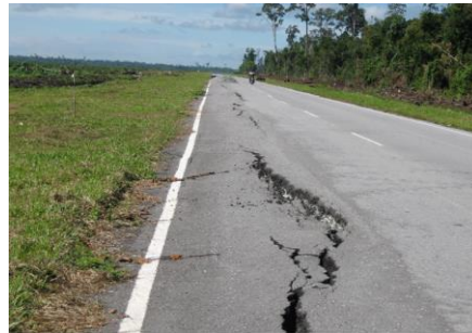
Figure 4. Damage to the road pavement due to surrounding peat area with ground water lowering. [3]
