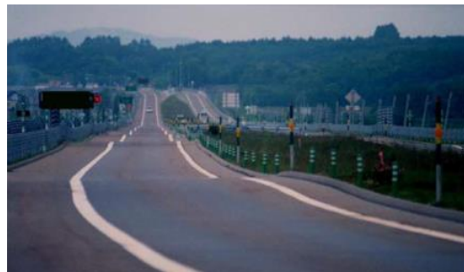
Figure 5. Long-term non-uniform settlement of road on peat ground. [31]
