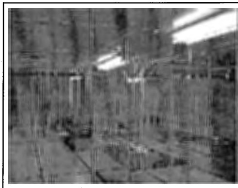
Figure 2: Cleanroom Plenum (negative) with Fan Filter Units.
